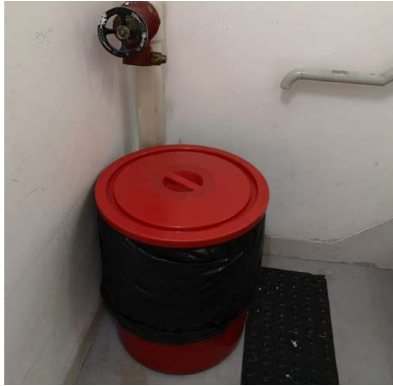
Trash bins squeezed into exit stairwells
