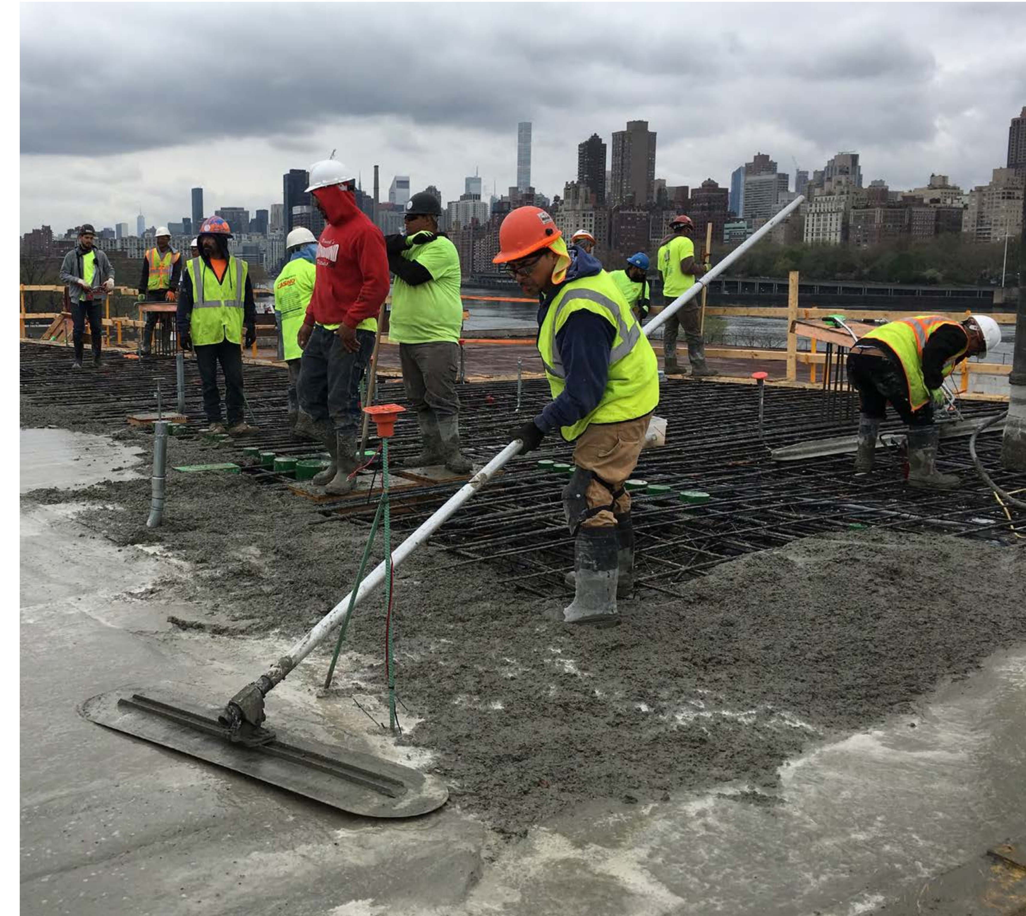
Pilot pour using concrete containing glass pozzolan as a cement replacement, Halletts Point NYC.
