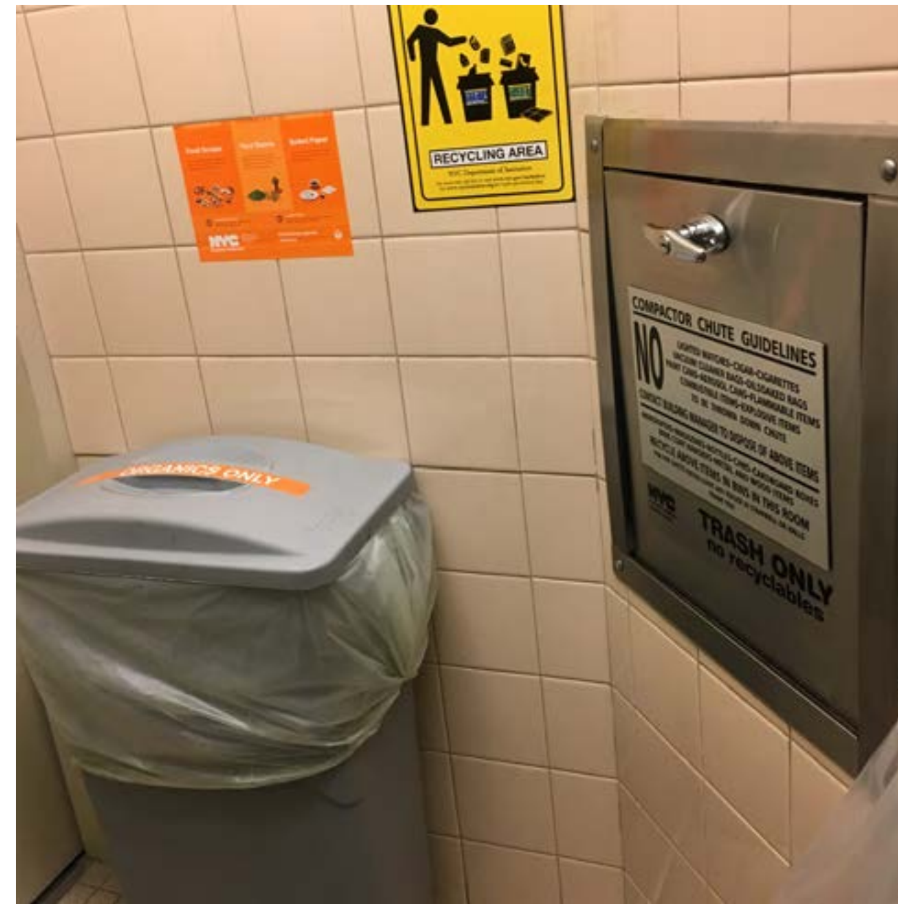
Organics bins may be in refuse rooms or central location
