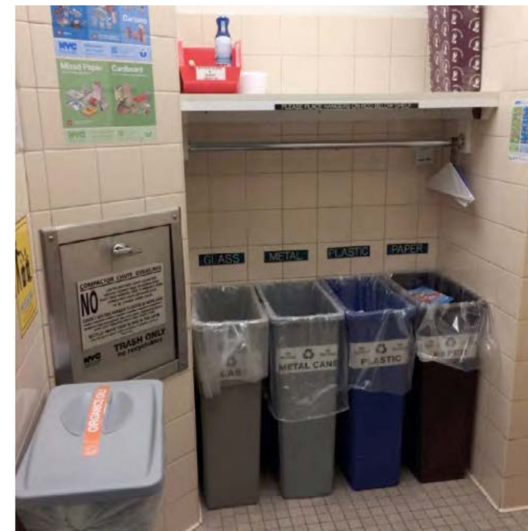
Equal convenience for food waste, recycling and trash via a chute in a waste room on every story of a NYC luxury building is convenient for residents.
