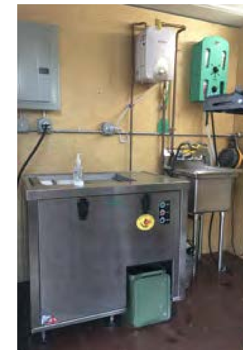
Pulper, utility sink, and hot water heater.
