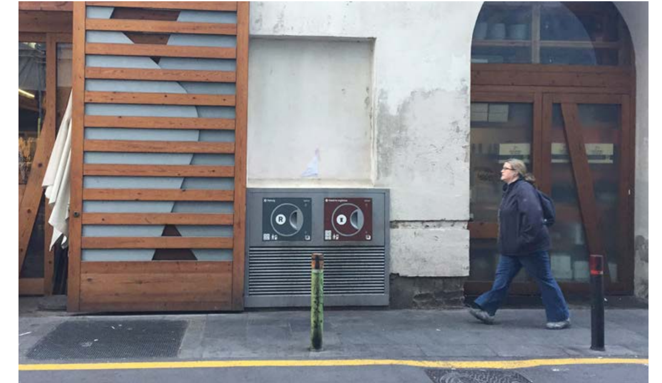
Pneumatic waste input points integrated into street wall, France.
