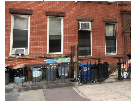
Waste in front yard areas can be unsightly, and likely causes odors for residents in ground floor apartments.
