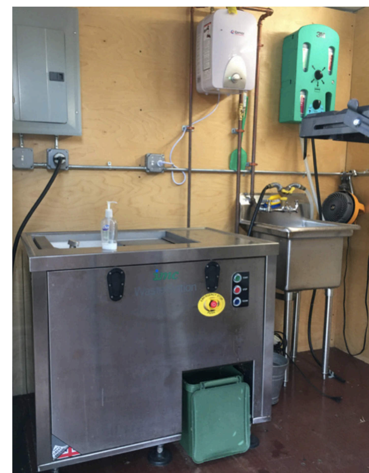
Pulper, utility sink, and hot water heater.
