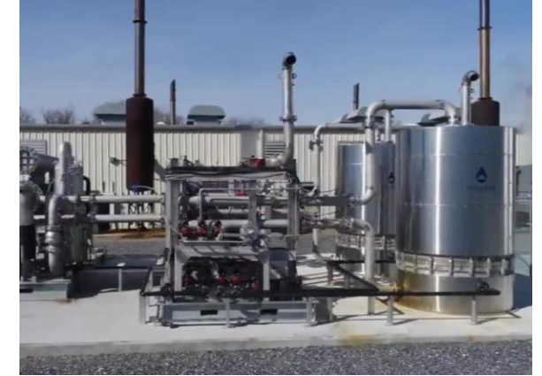
Granite Fuel RNG Upgrading Skid Photo credit: Granite Fuel
