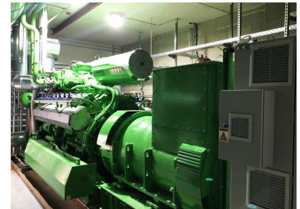
Jenbacher Cogeneration Engine Photo credit: Innio
