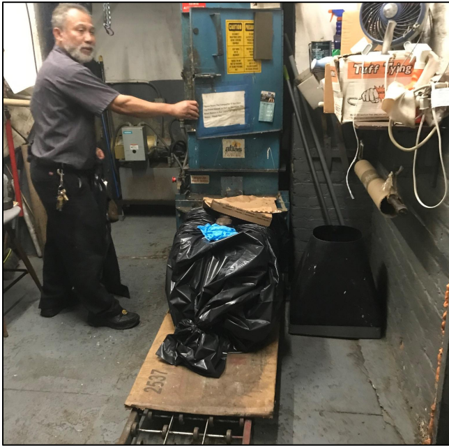
Chute compactors in NYC feed into a long plastic tube, and building staff need to cut and tie them into “sausage bags”.
